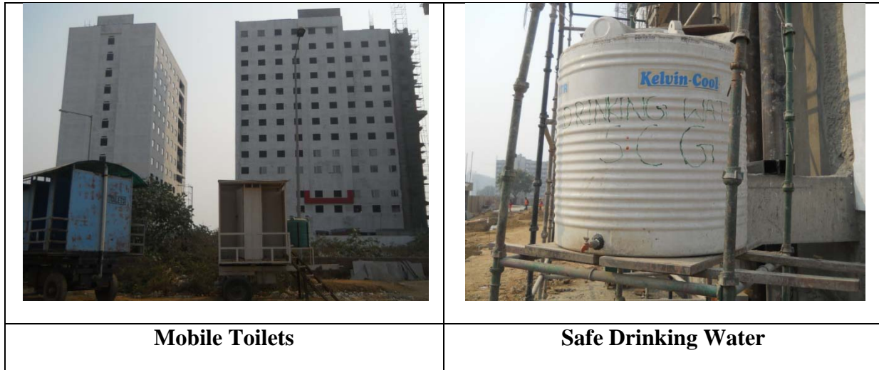
Figure No. 2 : Photograph of Mobile Toilets and Safe Drinking Water
