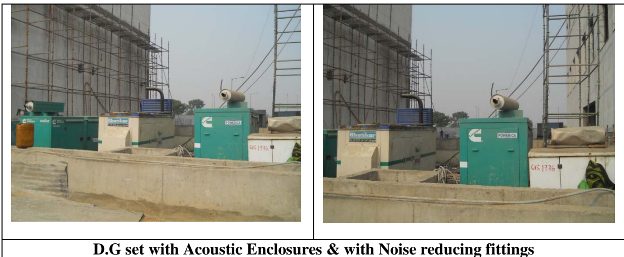
Figure No. 3 : Photograph of D.G. Sets
